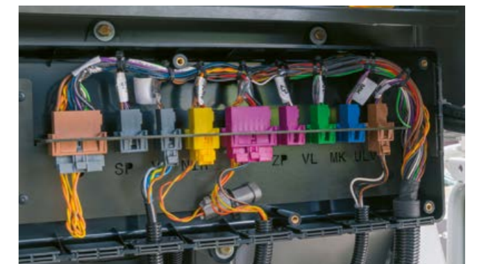
Expansion box in maintenance compartment
