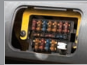
An accessible, compact fuse box for easy inspection
